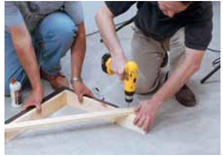
Fig. 3 BRACES. Before attaching the diagonal braces it's a good idea to make sure the bracket is square. Although you can build the brackets by yourself, the job will go much faster with two pairs of hands.
