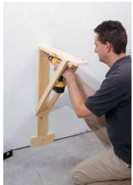
Fig. 6 ONTO THE WALL. Paul is attaching his brackets with 3" drywall screws into the wall studs. The small trim piece at the base of the bracket serves as a guide for how far from the floor the brackets should be, as Lionel will finish the room off with 3" trim.
