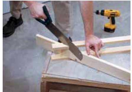
Fig. 4 AN EASIER WAY. Rather than trying to cut your angles before attaching the diagonal braces, it's much easier to cut the braces with a sharp hand saw after they are attached.
