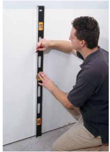
Fig. 5 GUIDELINE. A&LS operator Paul Burgess uses a four-foot level to draw a vertical line as a guide for attaching the bracket to the wall.
