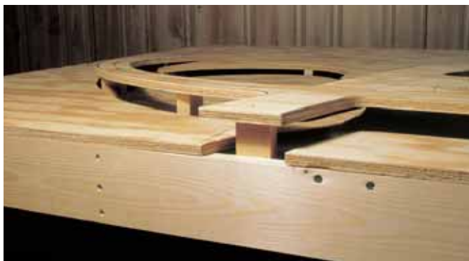
Fig. 4 RISERS. The 1 x 2 risers are in place under the road and railroad subroadbed. The lake area has been dropped down by notching the joists in that area.
